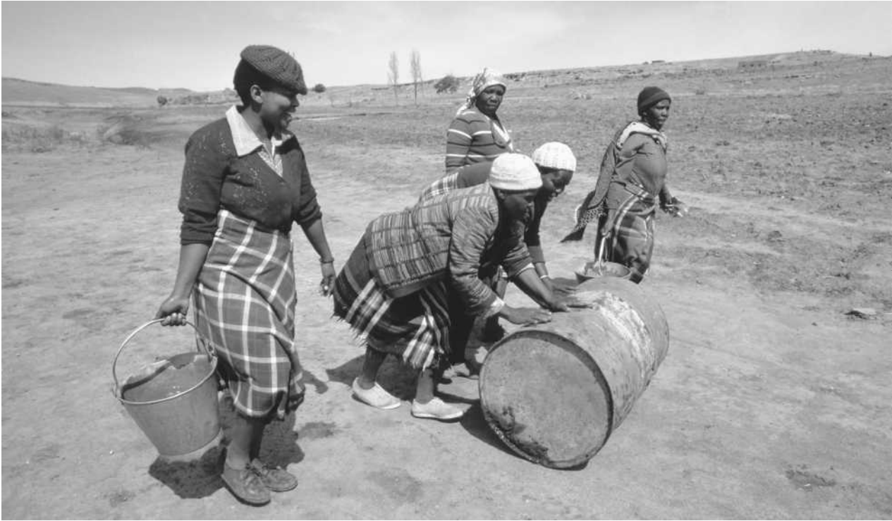
Women roll barrels and carry buckets containing materials needed for the construction of a reservoir.
